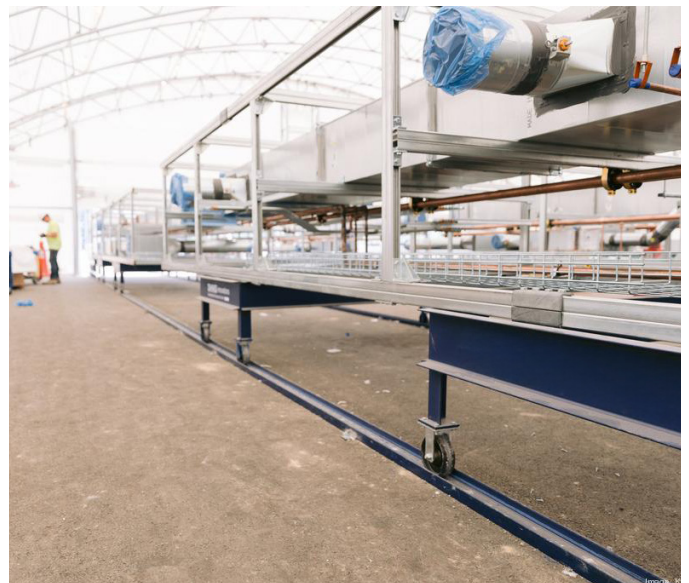
FIGURE 3: Prefabrication of MEP/FP & T ceiling racks can occur onsite/offsite with extreme precision, allowing Cable Tray to achieve the needed clearances for standards-based installations.
